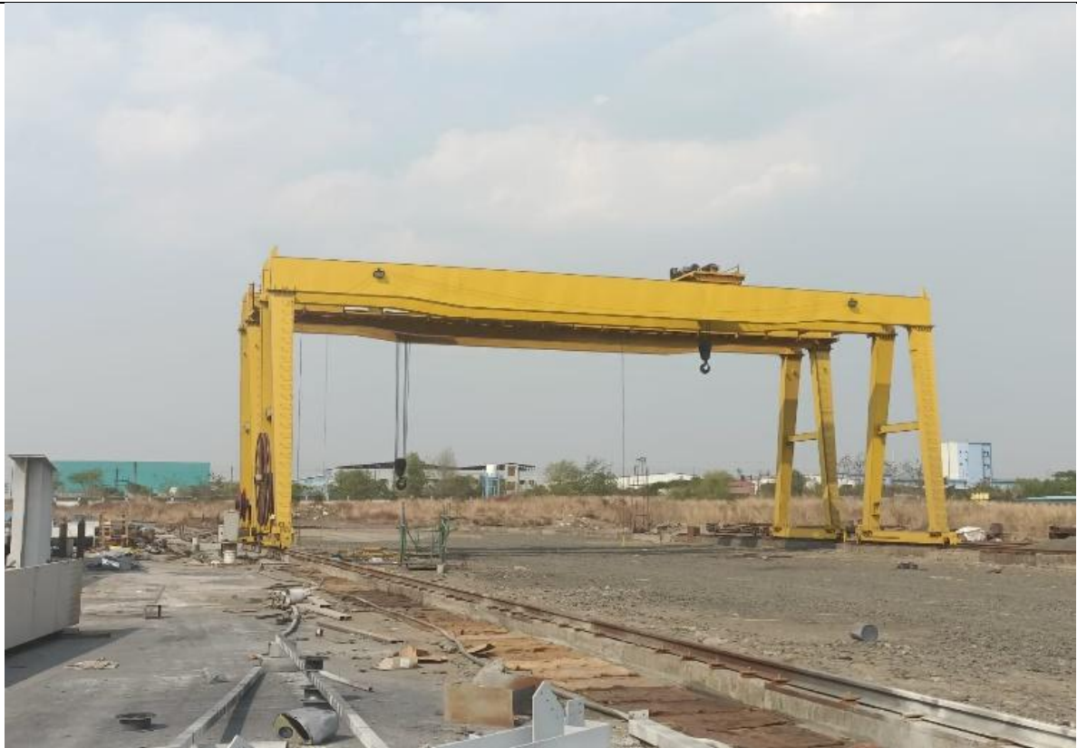
EOT CRANE-25MT CAPACITY
